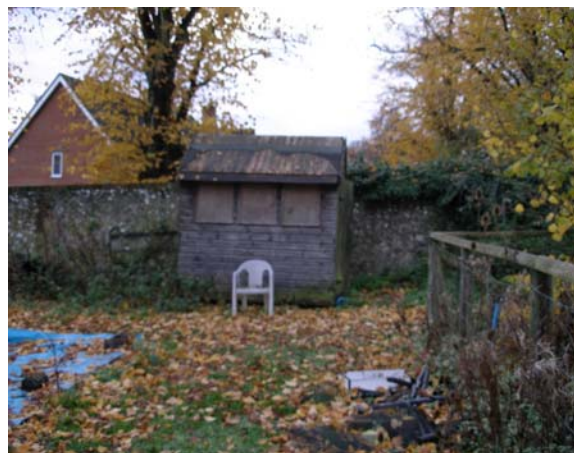
... hide roof in disrepair
